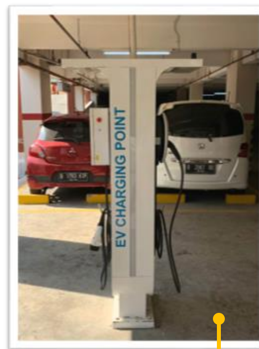
Commercialized Private Charging Apartment
