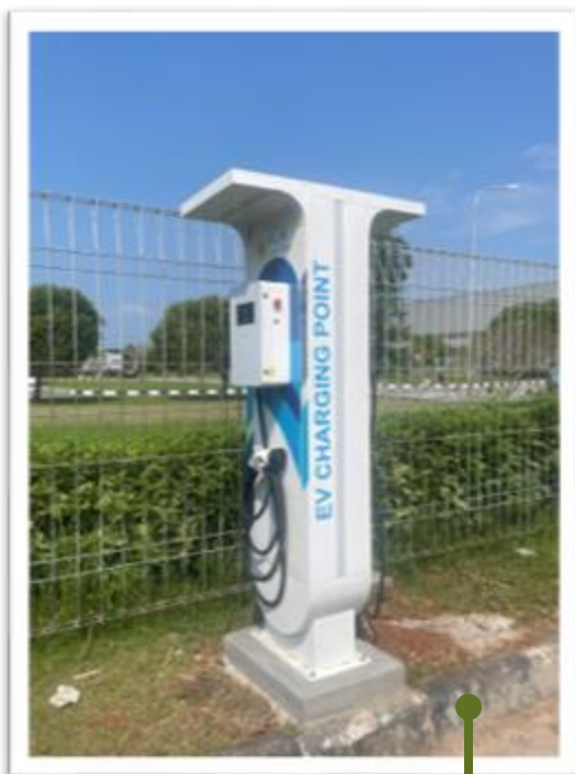
Private Charging in Manufacturing Site
